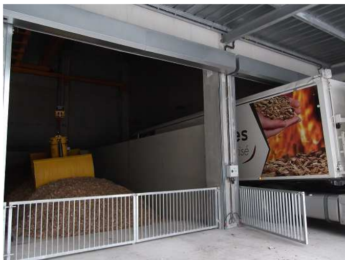
Stockage biomasse ©MRN
